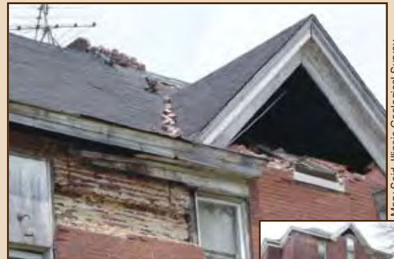
A wider view of the 1904 Berry School, Mt. Carmel, Illinois, shows the collapsed chimney, bricks missing from the wall, and bricks missing from the A-frame.
